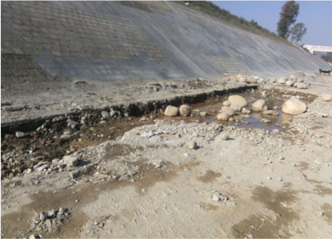
D/S of Asan Barrage Channel bed Near Bridge No 2 before start of closure work
