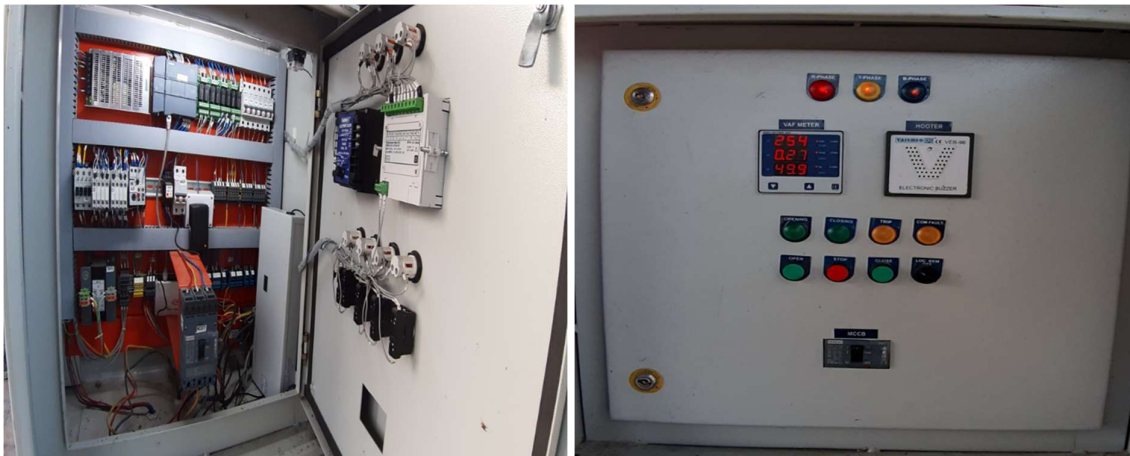
Local Panel for gate operation
