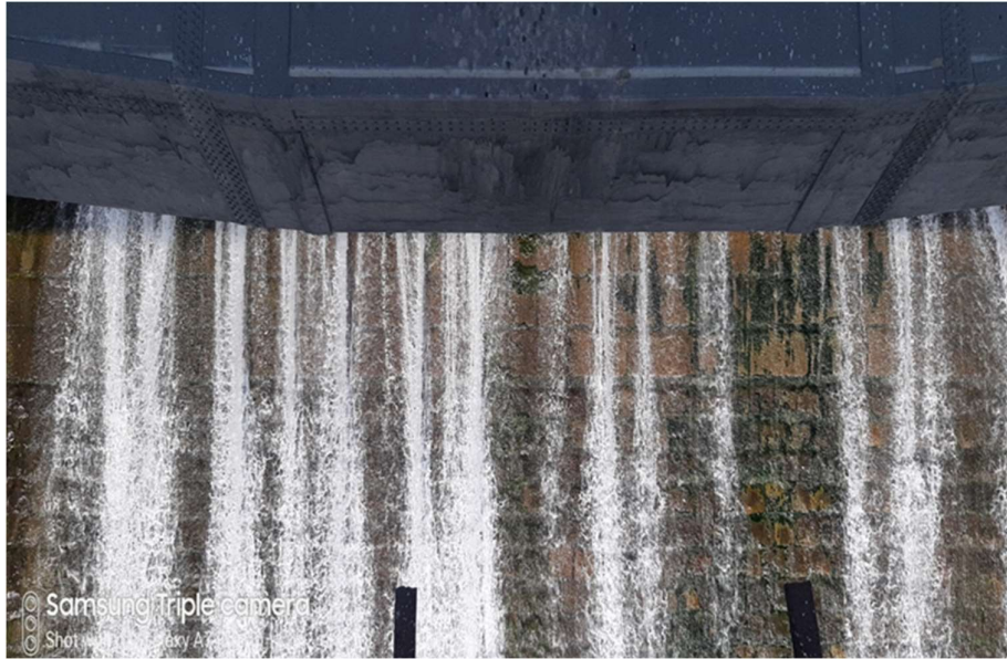
Barrage Gate before bottom seal replacement
