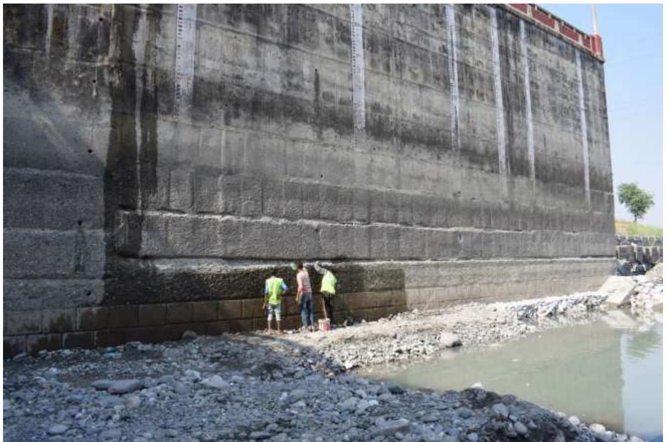
Status of abutment at gate no 1 before repair works at downstream
