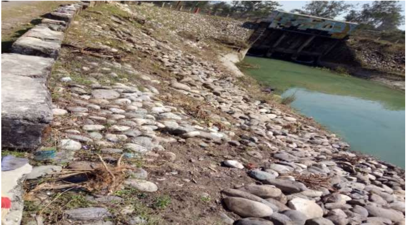
Status of right bank of silt ejector channel before repair works
