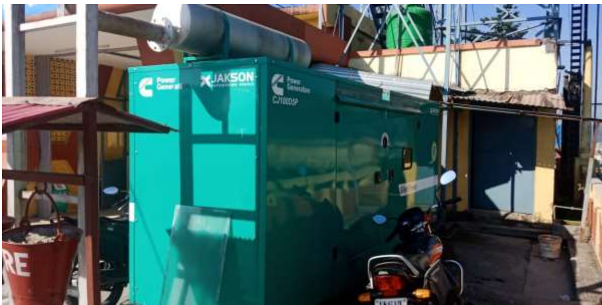
D.G. set (100kVA) after installation
