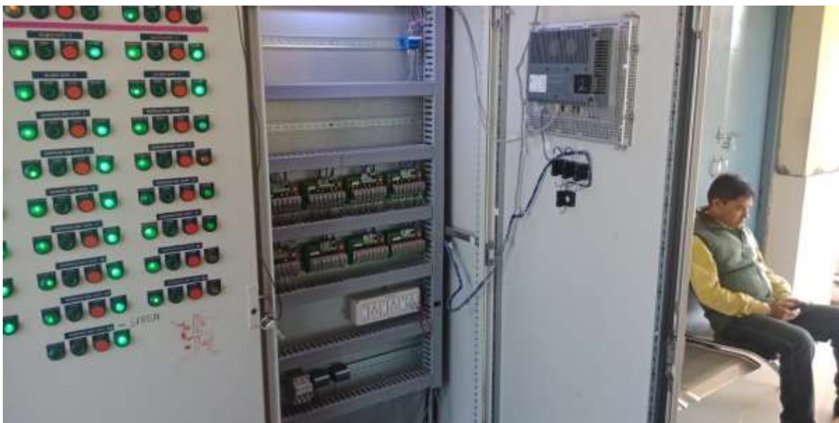
Barrage gates autmation system after installation
