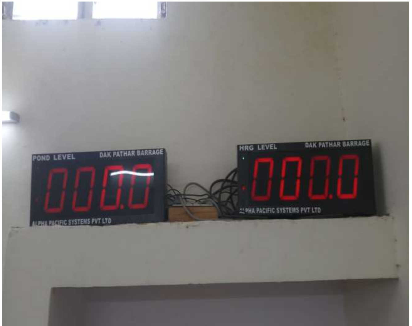
Remote Display of the Barrage Levels
