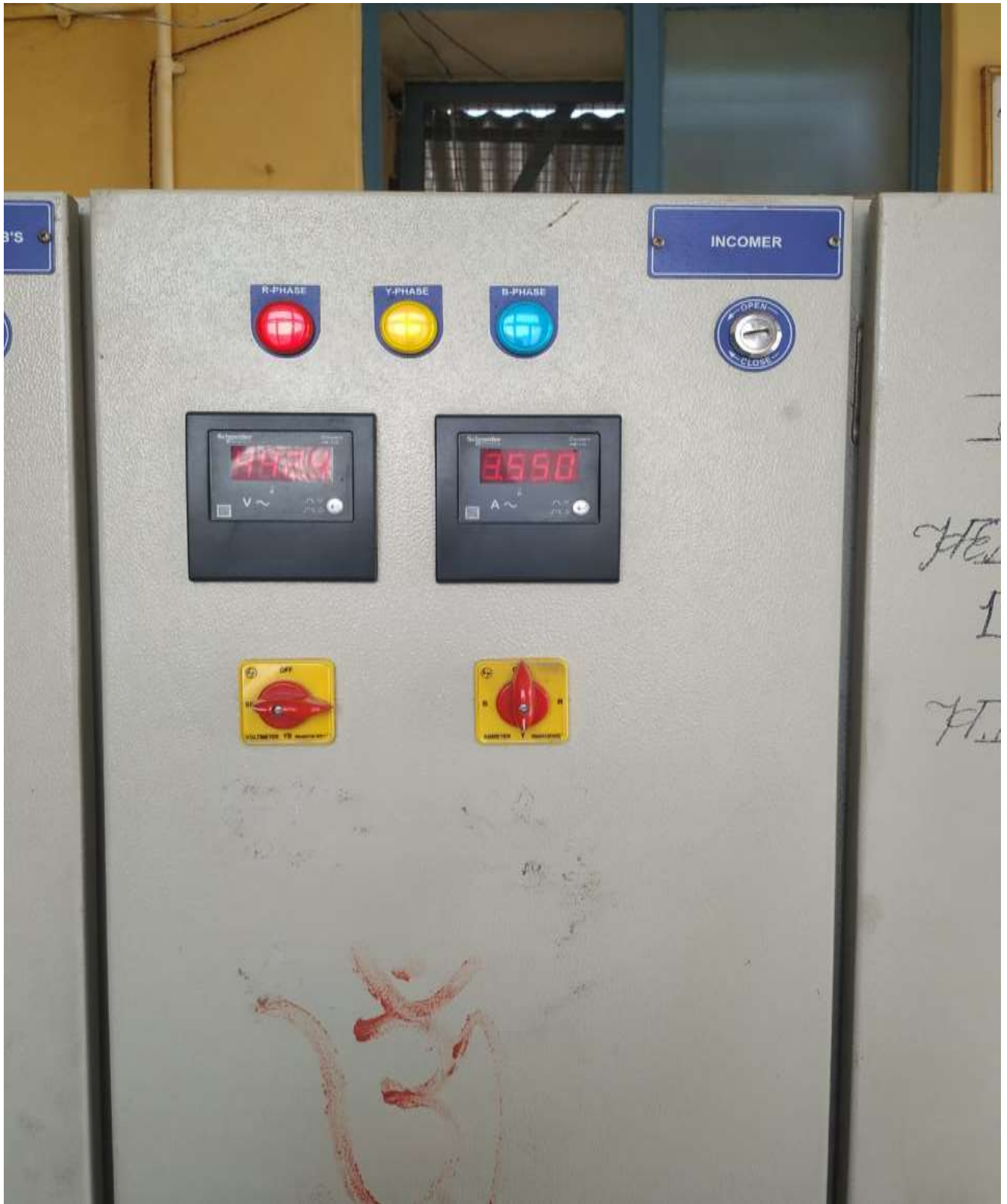
Power Supply Incoming Panel
