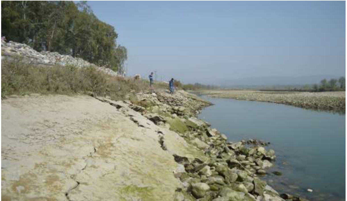
Status of upstream right bank before repair works
