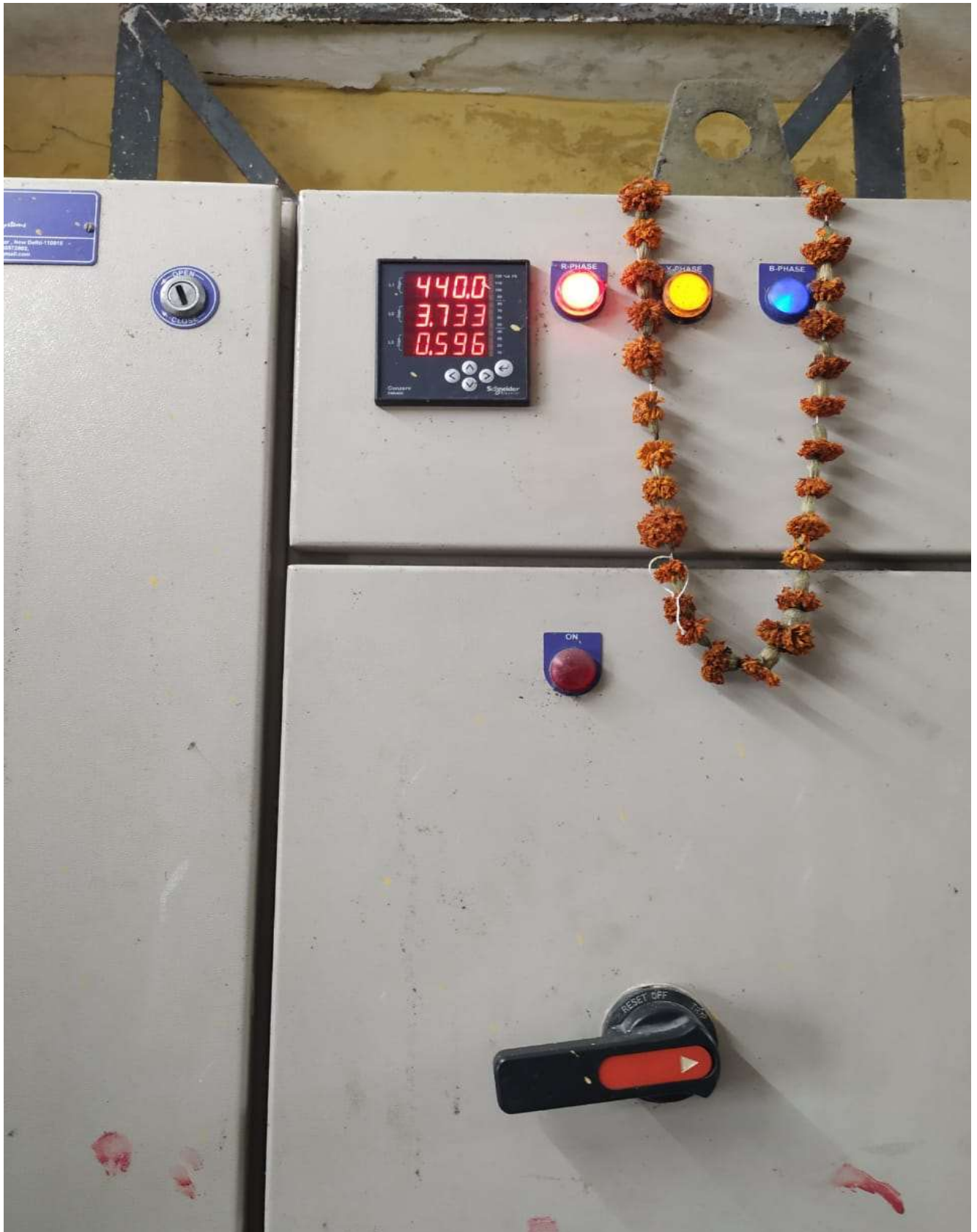
L.T. Supply Distribution Panel
